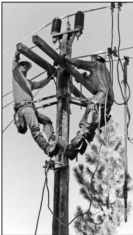
Above, Oregon Trail Electric Cooperative linemen work on lines from atop a pole. Photo by Steve Schauer. Opposite page, a Central Electric Cooperative lineman does some hot-stick work from a bucket truck. Photo by Jim Crowell.
