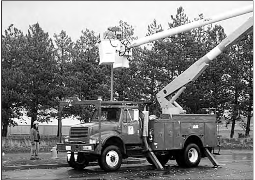
Klickitat PUD Groundman Mike Purdy checks on the progress of Lineman Martin Taylor and Foreman Rob Rising as they install a new light fixture in the PUD office parking lot in Goldendale.
