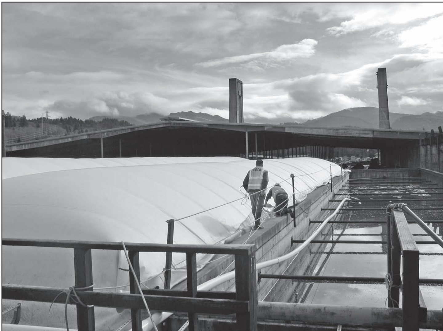
Workers at the Tillamook Biogas Facility in Tillamook, Oregon, check the Hooley Digester, which processes dairy manure and turns it into electricity and compost fiber. Photo by Dorene White, Tillamook PUD.
