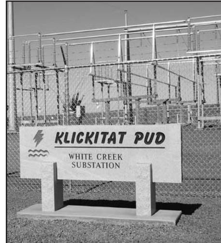
KPUD's new White Creek Substation.
