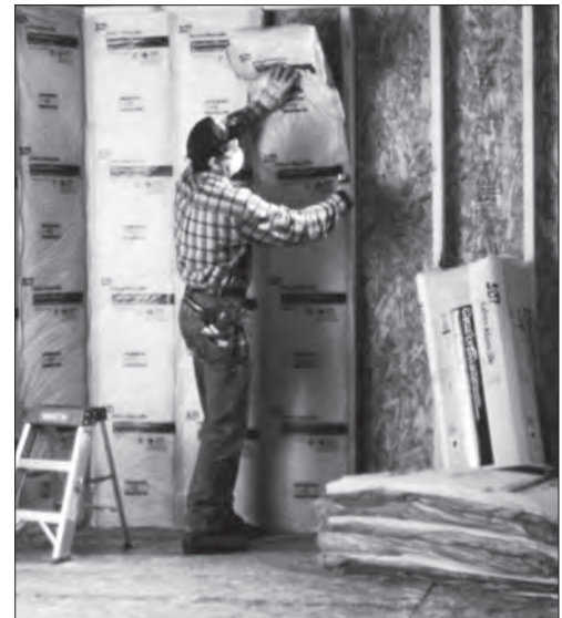
An R-value of 38 is recommended for attic insulation.
