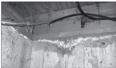
Use expanding insulating foam to seal wiring holes and gaps where the sill plate rests on the foundation.
