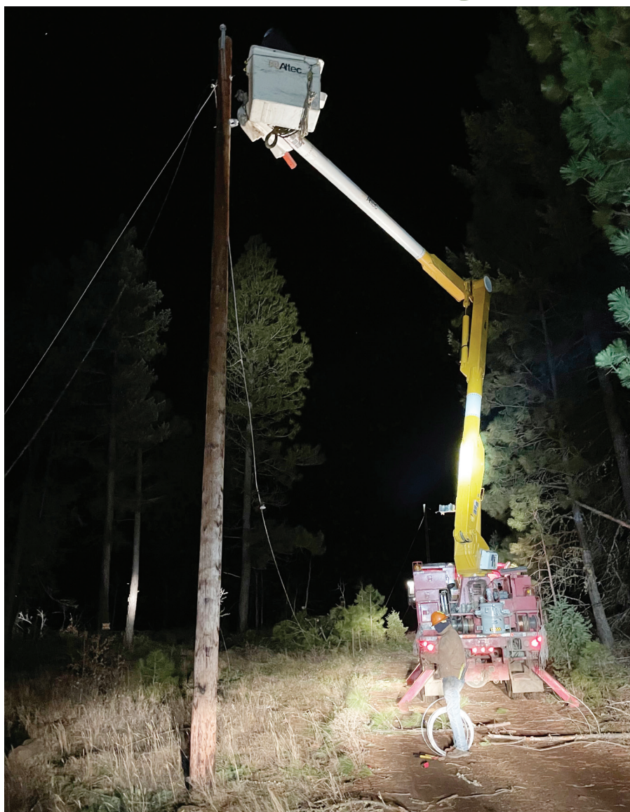
Klickitat PUD crews work to repair lines on England Drive near Box Canyon Road during the windstorm February 6. PHOTO BY GREG FAHLENKAMP
