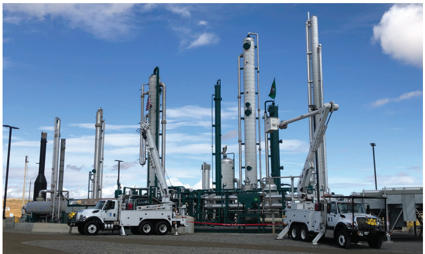
ABOVE: The H.W. Hill renewable natural gas facility produces more than 18 million gallons of renewable transportation fuel a year. OPPOSITE PAGE: White Creek is the largest public power-initiated wind project in the United States. Klickitat PUD owns a 13% share of the 68 average megawatts output annually. PHOTOS COURTESY OF KPUD
