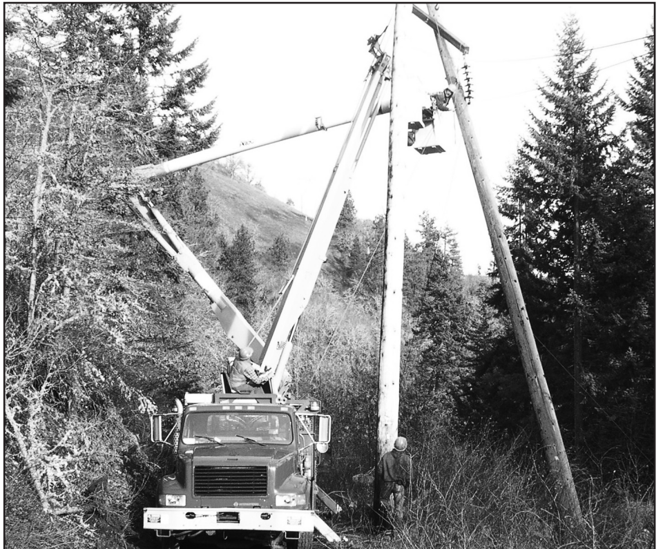
Above and top, KPUD crews were finally able, with help from Northern Wasco PUD, to restore all power by December 20. One KPUD lineman was injured when he fell down a pole.
