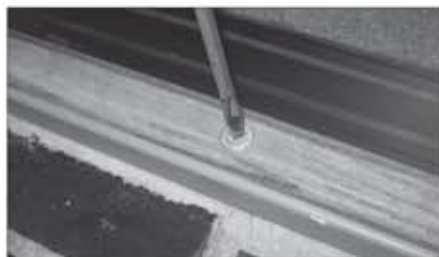
The threshold under the door can be raised or lowered with a screwdriver so the door bottom weatherstripping seals tightly.
