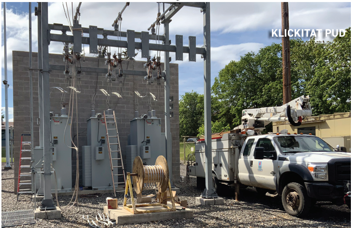
The Bingen Substation has been modernized through the years, including a recent installation of regulators to support the 2017 transformer addition.
