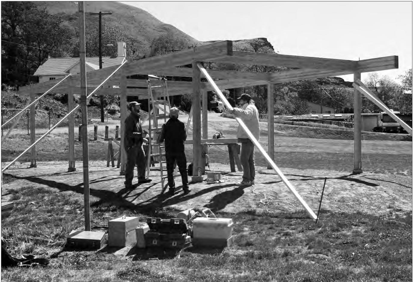
Jordan Harpole, left, Jack Bryant and Norm White raise a pavilion at the green space next to the Lyle Activity Center, former site of Lyle Elementary School.
