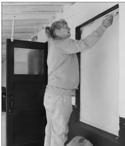
Volunteer Colleen Hatfield paints the outside of the old Lyle Elementary School, which has been converted into a community activity center.
