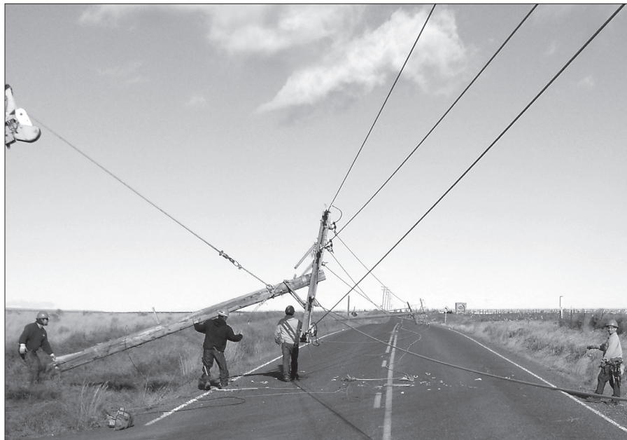
A storm in February 2008 knocked out power for approximately 12 hours while crews repaired multiple broken poles that snapped off in the severe wind.
