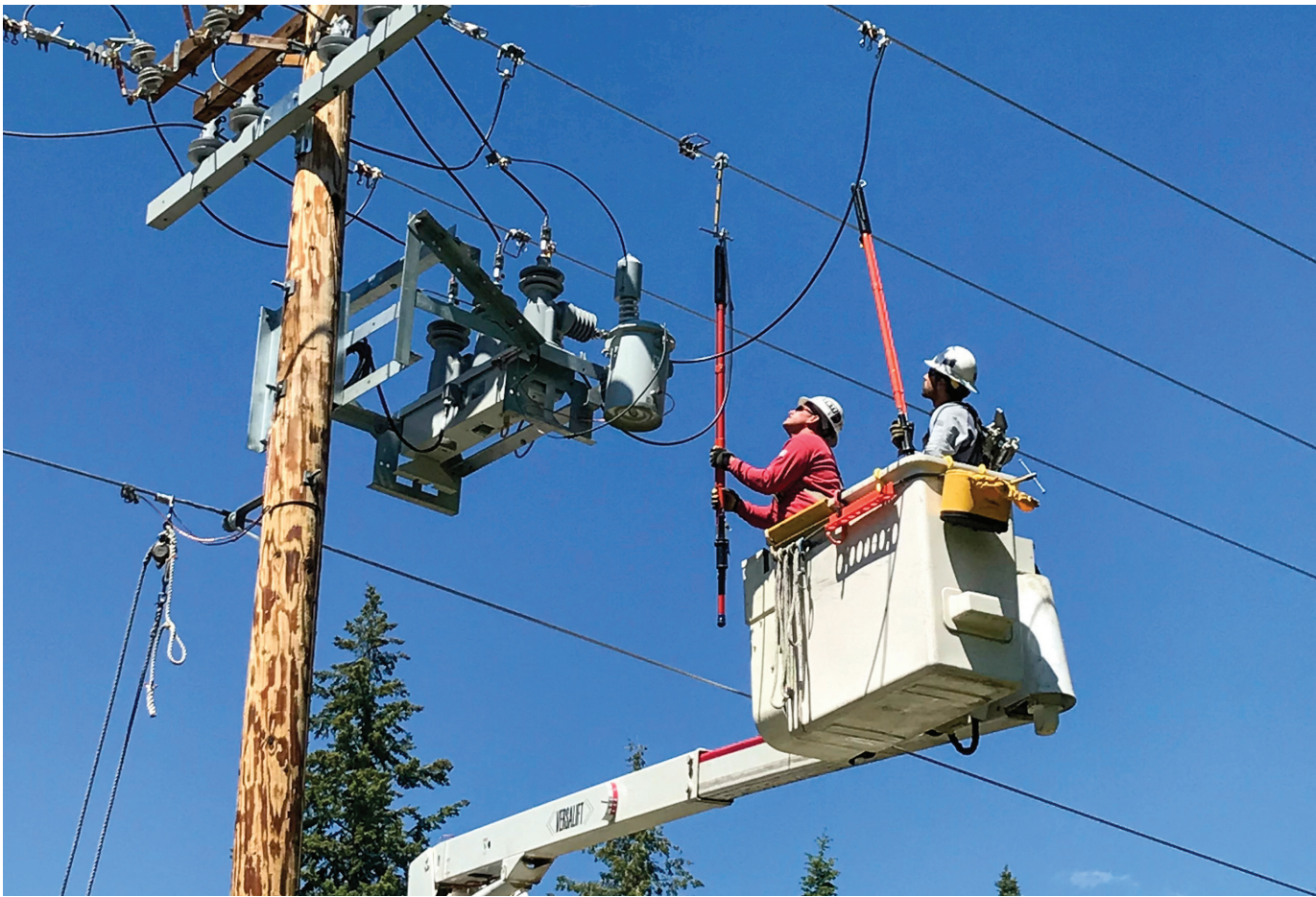
Turning off reclosers during the summer helps utilities prevent power lines from sparking wildfires. PHOTO COURTESY OF UMATILLA ELECTRIC
