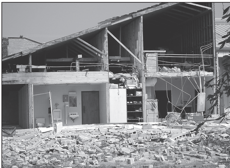
Above , only a partial shell remains at the Washington-St. Tammany Electric branch office in Slidell, Louisiana. Photo by Billy Gibson, Association of Louisiana Electric Cooperatives. Opposite page , an aerial view showing the aftermath of Hurricane Rita. Photo by Claude Ledet, Southwest Louisiana EMC.
