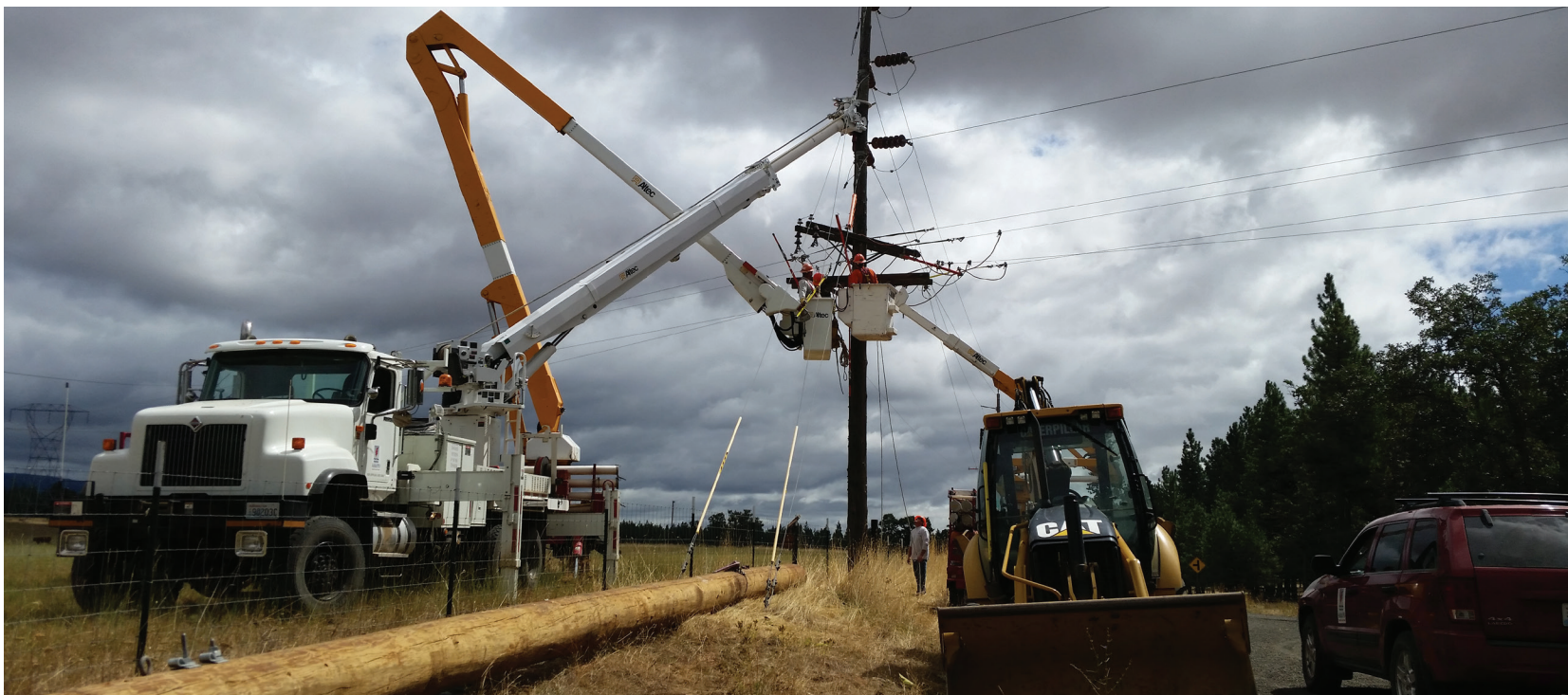
Crews work together to ensure you have safe, reliable electricity. PHOTO BY BRANDON JOHNSON
