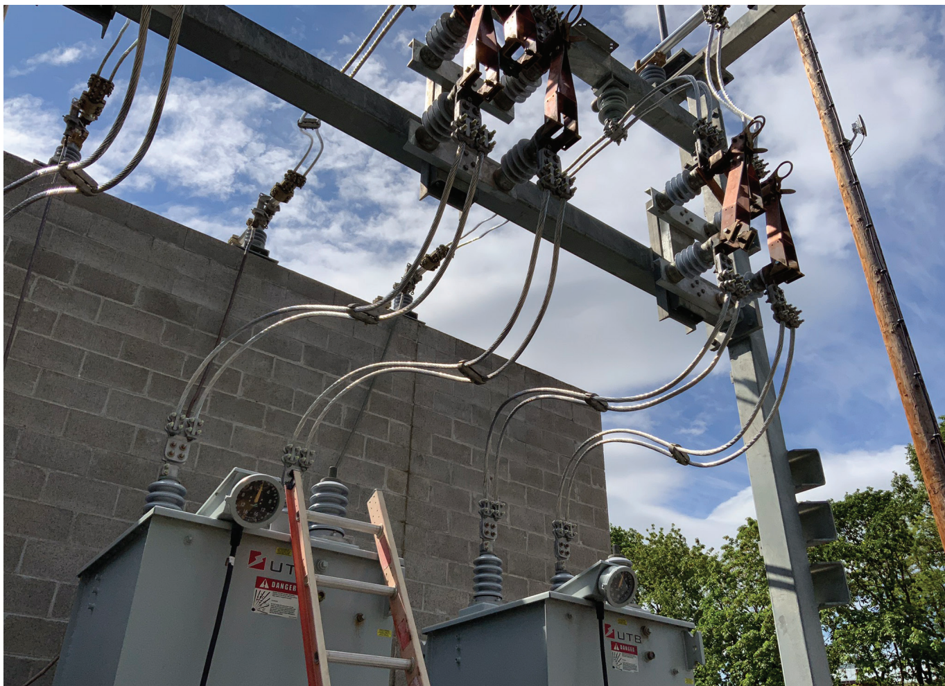
The Bingen Substation has been modernized through the years, including the most recent installation of the regulators to support the 2017 transformer addition.
