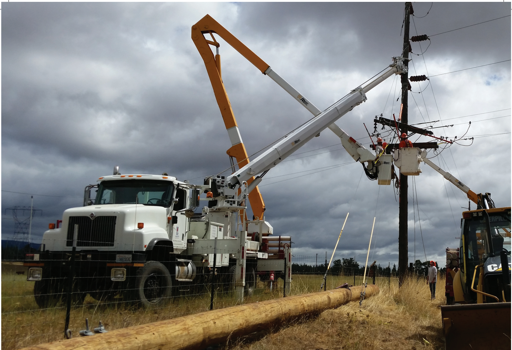
Crews work to ensure you have safe, reliable electricity. PHOTO BY BRANDON JOHNSON
