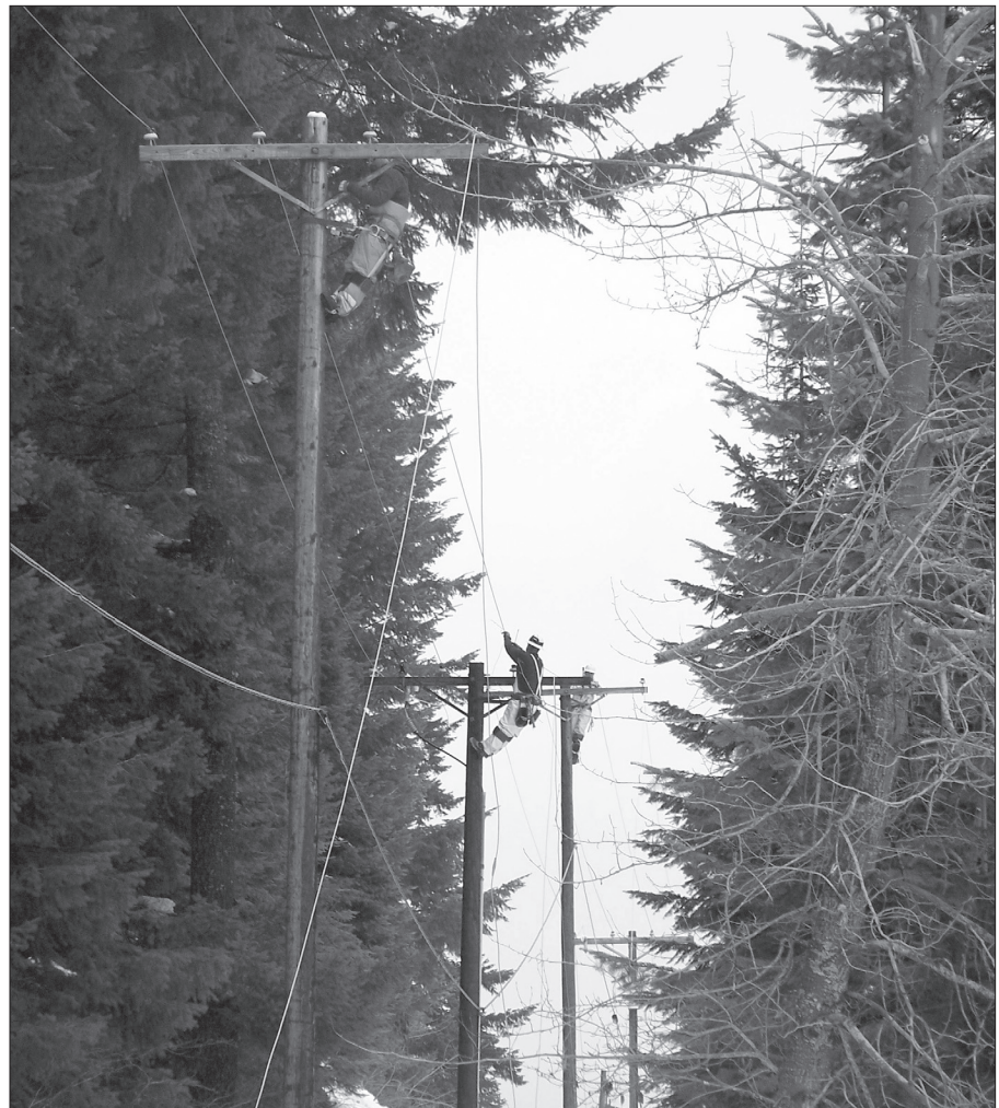
Klickitat PUD line crews work day and night to keep the power flowing to community homes and businesses.
